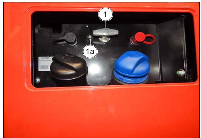
Figure 66: Battery disconnect switch
